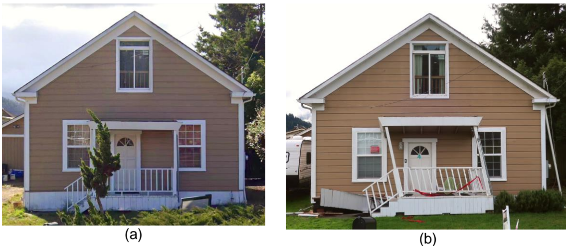
Figure 5.12. Home that fell due to failure of post-and-pier foundation system (east side is on left). (a) Before earthquake (undated Google maps street view image). (b) After earthquake. Home fell in the east direction. Notice tilting of porch posts and gutter downspout (at right) indicating large displacement of home.
