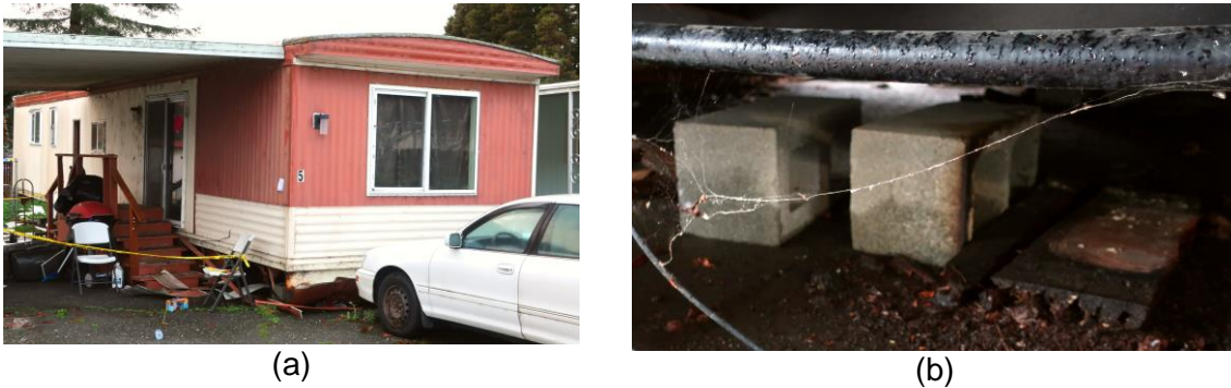
Figure 7.11. Collapsed home. (a) Home has dropped below staircase elevation. (b) View underneath home showing CMUs lying on their sides indicating that home was thrown a large distance to the east (to the left). Home did not have tie-downs.
