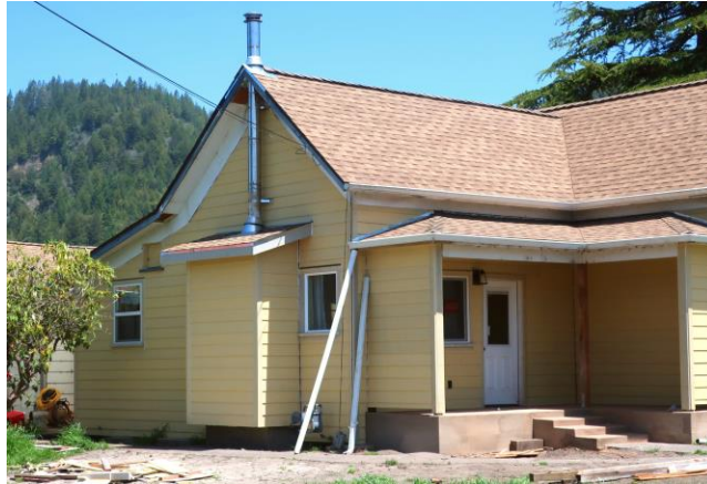
Figure 6.5. Home undergoing renovation in May 2023. This is the home that had its chimney tip over (Figure 6.3). The replacement chimney consists of a metal flue within a wooden enclosure. This is common chimney replacement practice.
