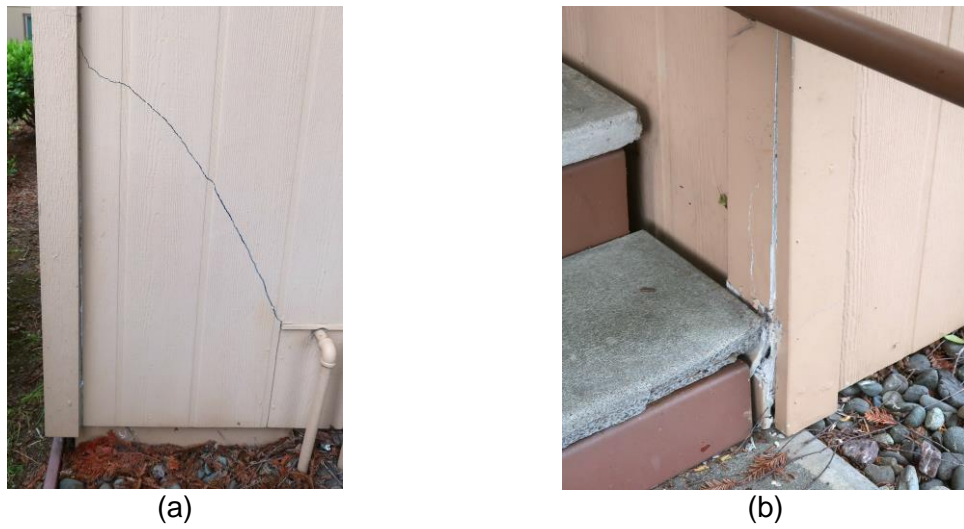
Figure 5.8. Examples of damage to rigid fiber-cement siding. Buildings had extensive siding damage. (a) Diagonal crack in siding. (b) Broken vertical molding.
