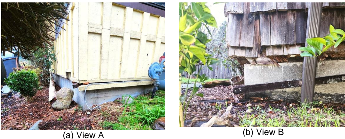
Figure 5.10. Close-up views of home showing offsets caused by earthquakes (Figure 5.9b). (a) View A (Figure 5.9b). Sill plate was split and home moved to the east at this corner (to the left). (b) View B. Sill plate was split and home moved to the south at this corner (to the left). Cripple wall above was also tilted to the south. There were some anchor bolts connecting sill plates to concrete foundation.
