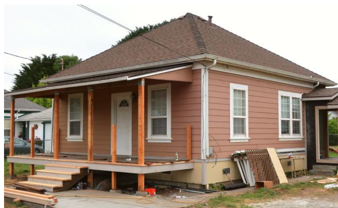
Figure 5.4. Home undergoing repairs in May 2023. This was the home that shifted off its foundation shown in Figure 5.2a. The home was lifted up and placed back on a new foundation.
