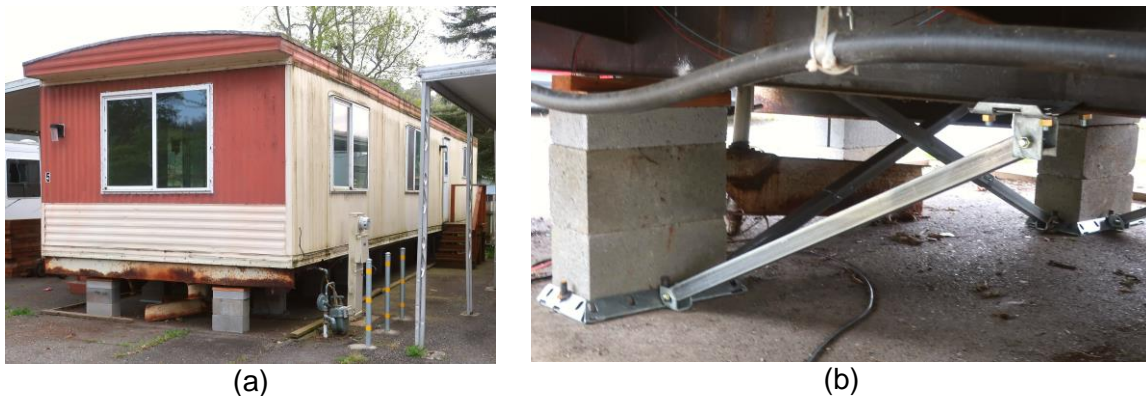
Figure 7.12. Home undergoing repairs in May 2023. This was the home that collapsed shown in Figure 7.11. (a) Home was lifted up and placed on piers with skirting yet to be installed. (b) View underneath home showing new bracing system.
