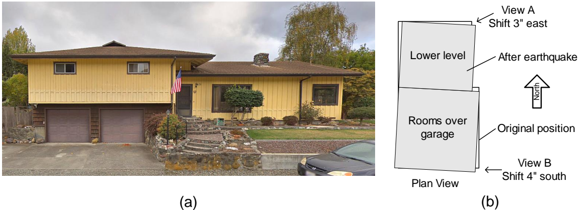
Figure 5.9. Split-level home that suffered damage. (a) Street view of home before earthquake (undated Google maps street view image). Home built in 1962. The upper level rooms over garage (on the left) are situated on stepped concrete footing stem walls with cripple walls extending from top of walls to floor elevation above. Cripple walls are shorter toward the back of garage. The lower level (on the right) has floor joists sitting on wood sill plates situated on top of footing stem walls (no cripple walls). (b) Plan view depicting shifting of home caused by earthquakes.
