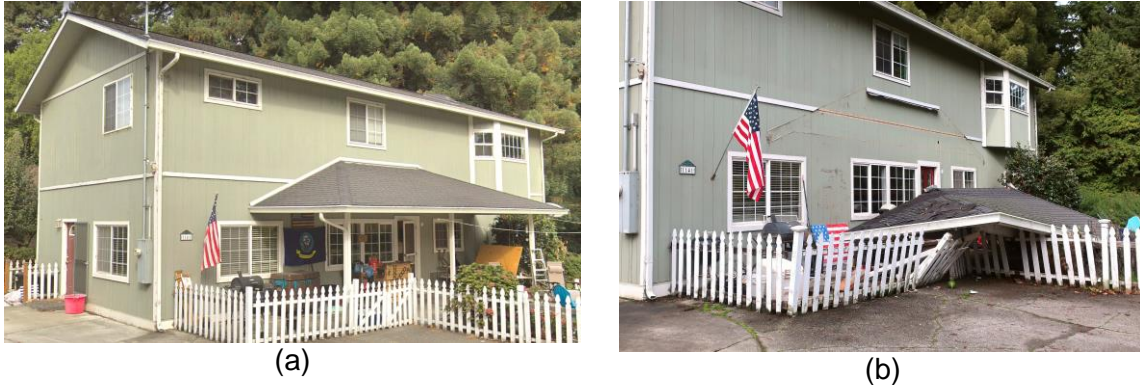
Figure 5.6. Example of home that suffered porch roof collapse (home built circa 2000). (a) Before earthquake (undated Google maps street view image). (b) View after earthquake with porch roof on ground and crushing fence.
