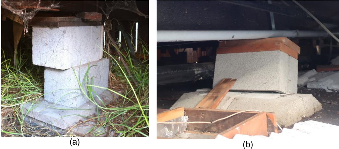
Figure 7.13. Views underneath damaged homes showing piers. (a) CMU pier that was offset (slid) between units. (b) CMU pier that slid on precast concrete pad and then tilted.
