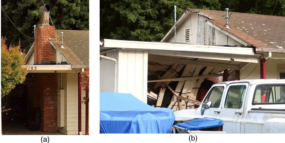
Figure 6.2. Example of masonry chimney collapse. (a) View before earthquake (undated Bing maps street view image). Home built circa 1935. (b) View after earthquake. Chimney collapsed and fell through attached carport roof. No signs of straps connecting chimney to home.
